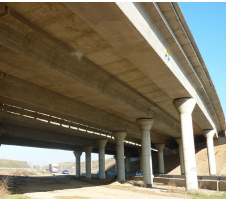
M-203 Highway - Viaduct over M-206 road (Madrid) - 3 narrow beams (1.50 m high) per span, supported by circular piers
