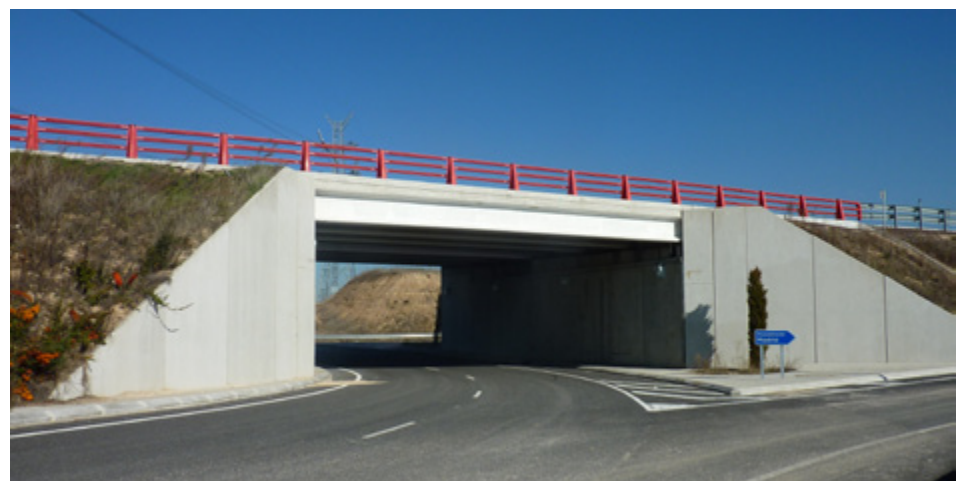
Pass under M-503 Highway (Madrid - SPAIN) - 8 IL-100 beams per span, supported by buttressed panel abutments
