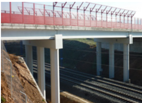
M-224 Road - Structure over high speed line railway in Torres de la Alameda (Madrid) 3 span deck, 4 IP-130 beams per span, supported by a portico, made up of 3 octagonal piers (9 m high) plus a lintel
