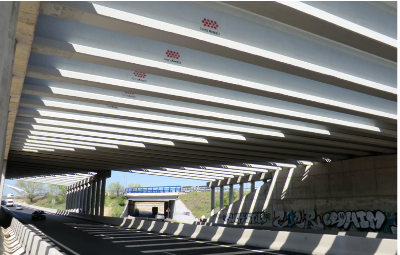
Connection from Torrejón de Ardoz (MADRID - SPAIN) to A-2 highway (Madrid - Barcelona)
