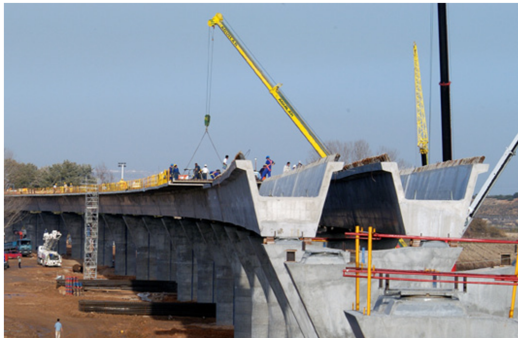
High Speed Train Viaduct - Section Mocejón - Toledo (SPAIN) - Spans length: 36 m - 2 narrow TA-260 beams per span
