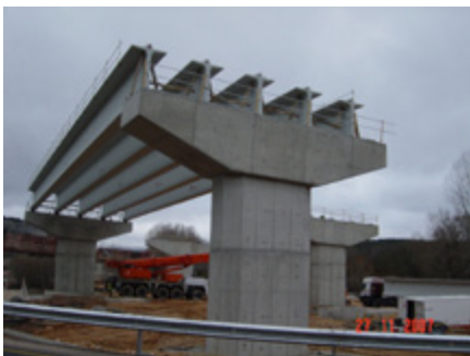
A-67 Highway (Palencia - SPAIN) - Section: Alar del Rey – Puebla de San Vicente - Viaduct 2.9 Solution: 5 IP-200 beams per span
