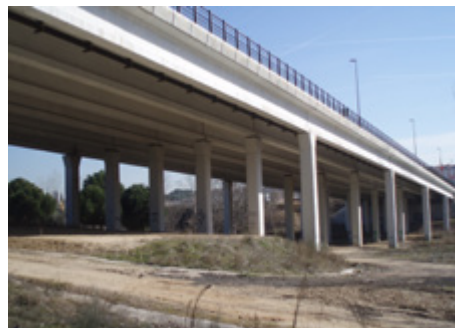
Viaduct over the Combos river, in Arroyomolinos (Madrid - SPAIN) 6 span deck, 6 IP-165 beams per span, supported by square piers (9 m high) with bell capital, without lintel
