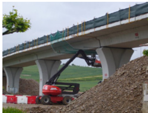
A-12 Highway (Camino de Santiago Highway) - Herviás-Grañón section (La Rioja - SPAIN) - Overpass with wide TA-90A mono-beam, supported by palm shaped precast piers
