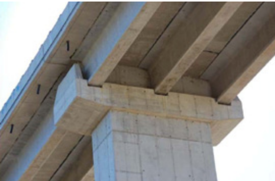
Seismic diaphragms between I beams to impede transversal movement and deck offset
