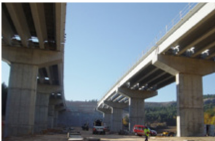
A-67 Highway (Palencia - SPAIN). Section: Alar del Rey – Puebla de San Vicente - Viaduct 2.3 Solution: 5 IP-155 beams per span
