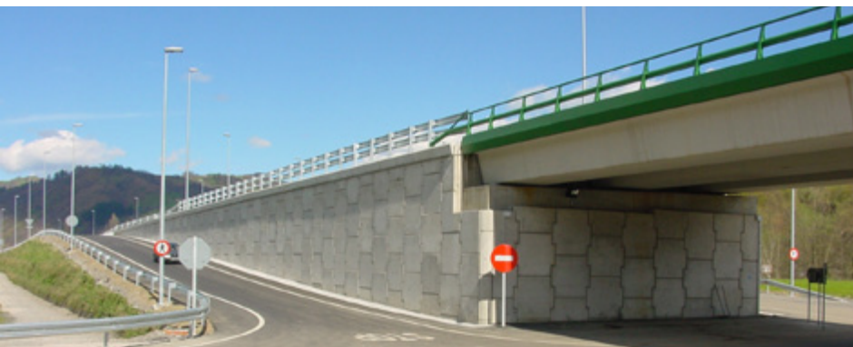
Pass under Corredor del Nalón road. Sotrondio – Barredos section (ASTURIAS – SPAIN) Reinforced earth abutment, supporting U beams
