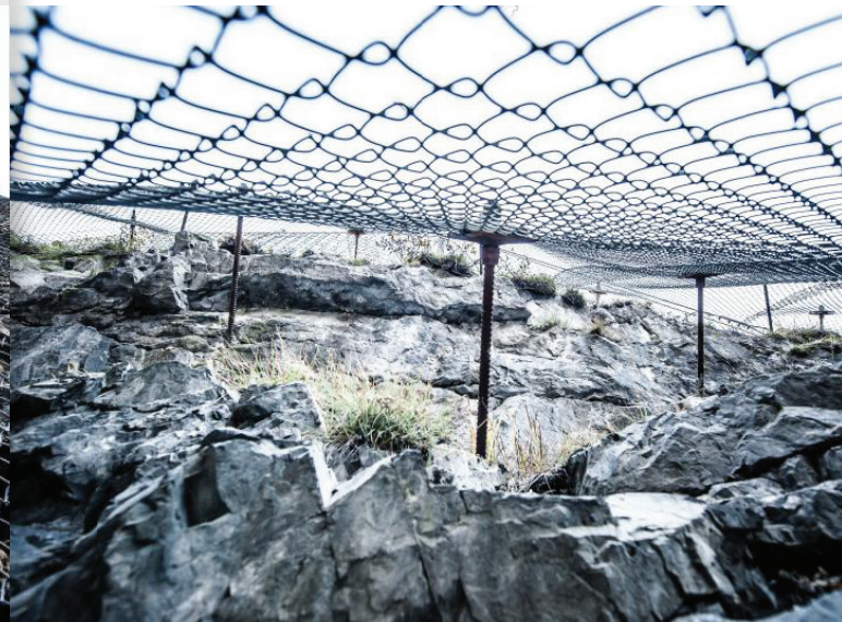
An example of a slope mesh system designed to protect a highway from falling ice that builds up on the slopes during the winter.
